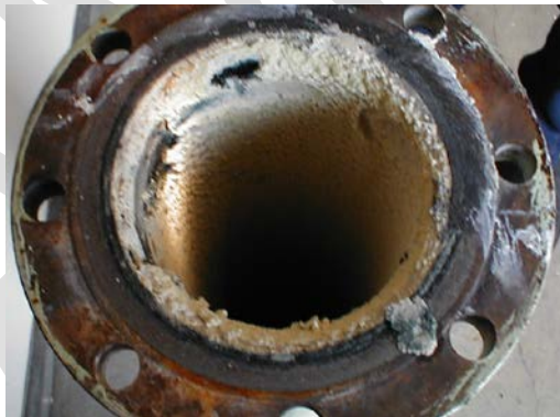
Figure 3-9 – Accumulation of Post-precipitation Scale on Cooling Tower Blowdown Line
