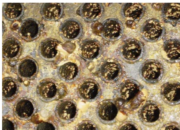
Figure 2 – Tubesheet of Carbon Steel Heat Exchanger
