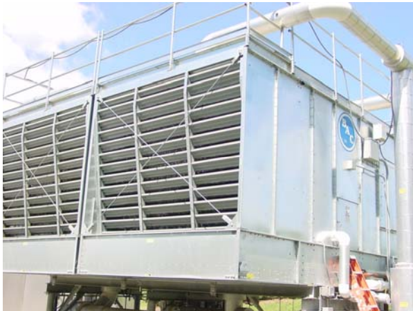
Figure 1 – New galvanized cooling tower
